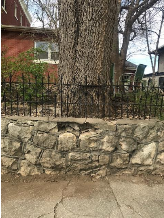
One of the major threats to the integrity of historic stone walls is the damage done by vegetation.
